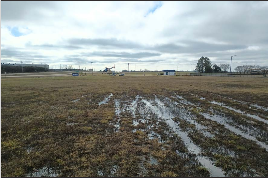
Figure 7. View of the standing water in the southern portion of the project area, facing south.
